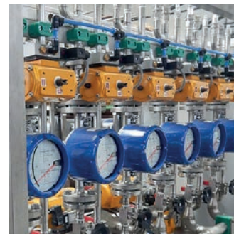
Energy from Waste – Adaptation of existing SNCR
